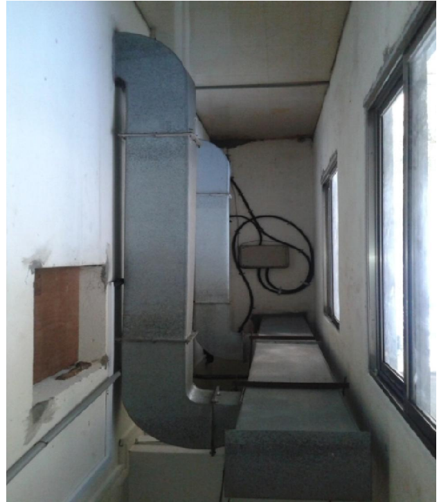
Exhaust system outlets
